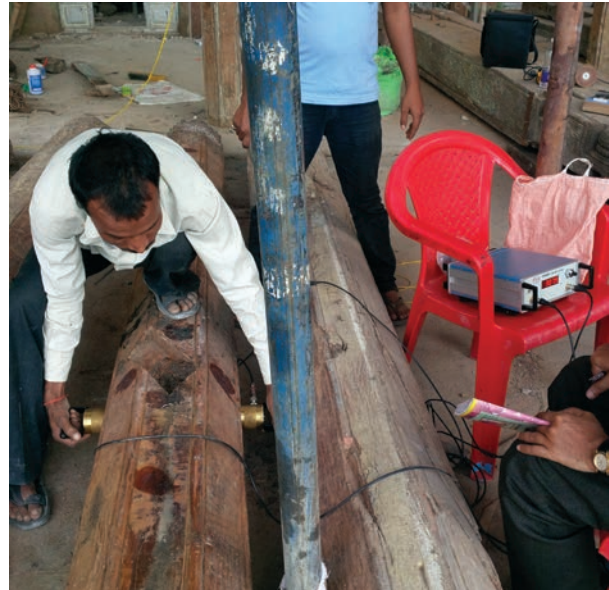
Testing timber using Schmidt Rebound Hammer. Source: Jeernodhar Conservators Pvt. Ltd. project in Gulbarga, Karnataka
