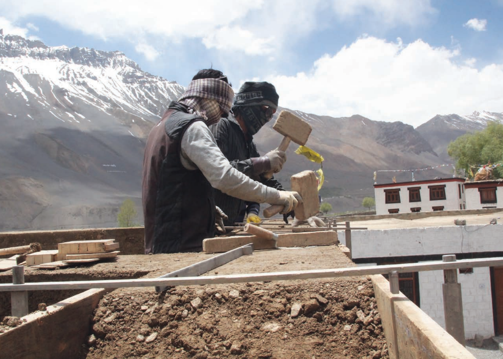
The rammed earth being compacted with hand-held mallets to allow air to remain within the soil mix
