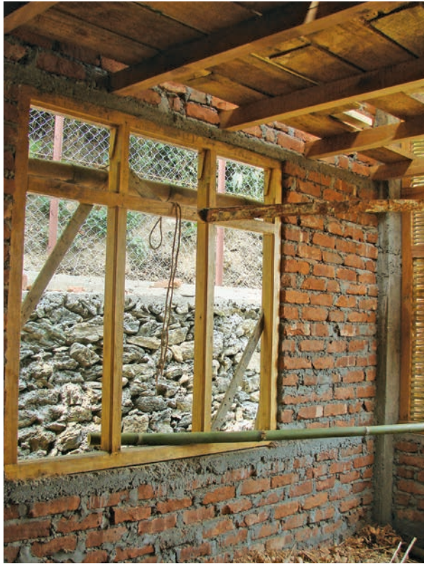
Window frame fixed in the wall on the backside of the cottage
