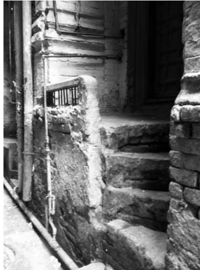
Entrance steps from sides along external wall in narrow streets for high plinth
