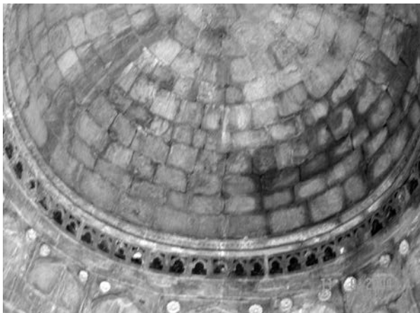
Tiles in miniature arches at interior of porch, Hoshang Shah's Tomb, Mandu
