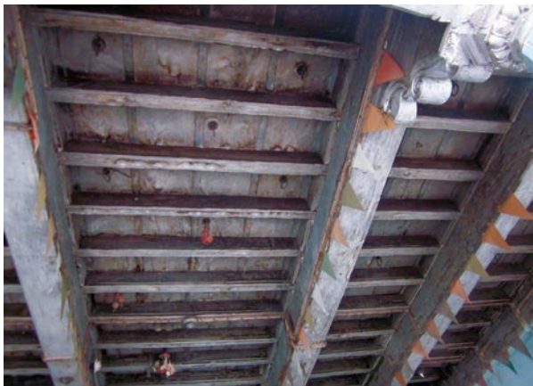
Timber restoration of roof structure, Ahilya Wada, Maheshwar, RGRA, 2005 with old and new timber using variety of joinery techniques
