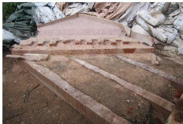
Process of construction/restoration of Madras terrace in layers: small bricks on edge, bricks laid flat and then lime concrete, etc. Source: RGRA project in Aneondi, Karnataka
