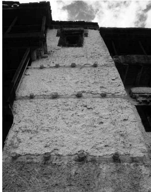
Floor beams resting on primary beams serving as wall plates, Chemrey Monastery. Source: Peeysuh Sekhsaria
